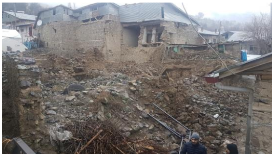
Fig. 5. Total Collapse of Adobe Structures in Sivrice Earthquake - Duygulu Village – Courtesy of Dilek Okuyucu
