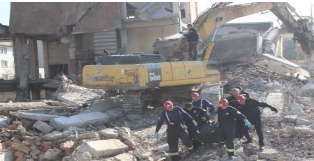
Fig. 1. The accident that occurred during the demolition
