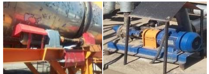
Figure 2. Electric motors in asphalt plant
