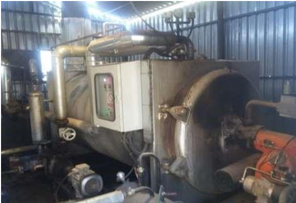
Figure 2. Hot oil boiler.
