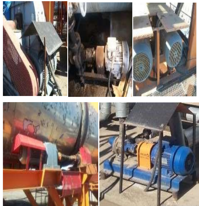
Figure 4. Electric motors in asphalt plant
